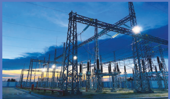
110kV substation of Wind Farm 7 - Phase 1 in Soc Trang province - a place with great potential for renewable energy
