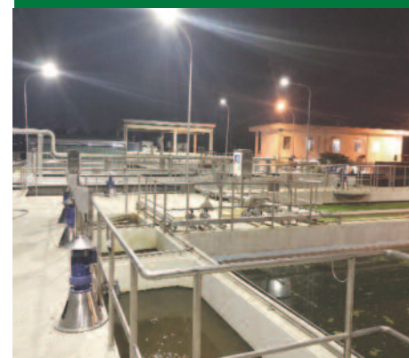
The centralized wastewater treatment system is modern and standardized
