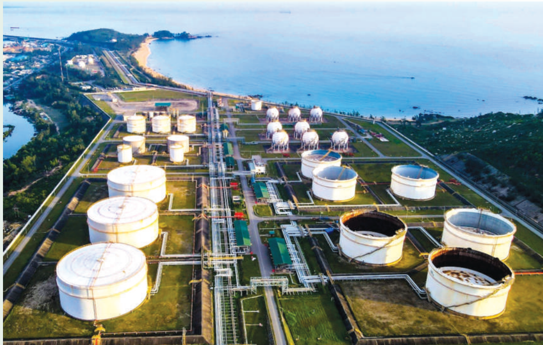
Maintaining refinery operations is a key task to ensure a stable fuel supply for production and daily consumption
